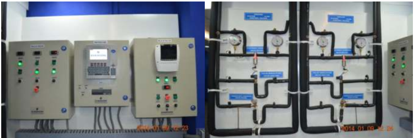
Advanced Refrigeration Controls/Remote Monitoring Systems
